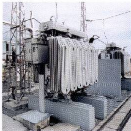
Jankovci - željeznički transformator
